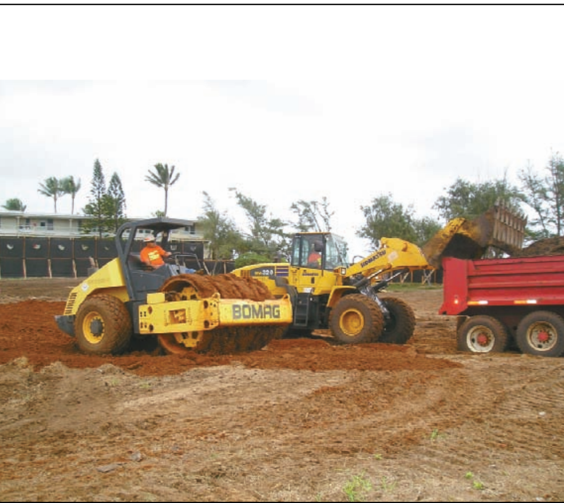
Construction started on the Waipouli Beach Resort in October. Bulldozers and trucks have been moving tons of dirt and, soon, the foundation will be underway.
