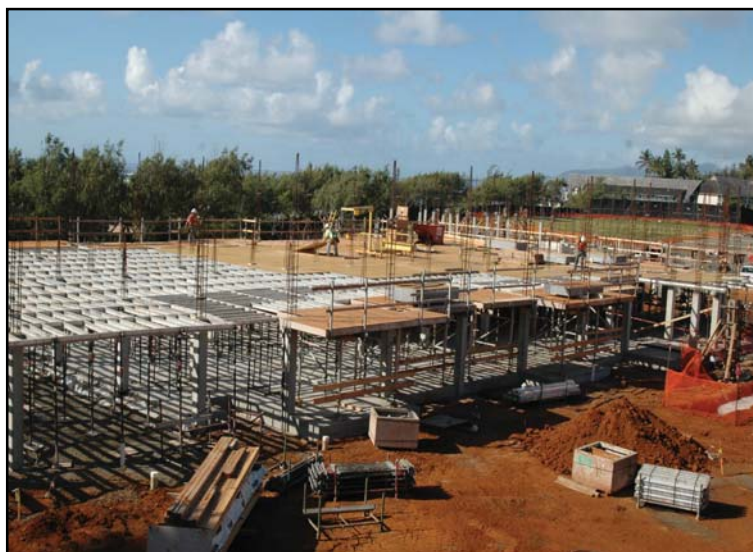
Going up: By May of this year, phase one and two of the resort was taking shape, including foundations and columns. Developers expect to complete the resort by the end of 2006.
